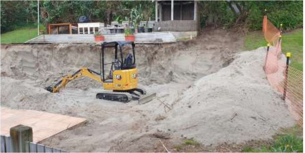
View of the western neighbour's backyard, with the hedge removed and temporary fencing about 4m into the Waikanae Church property.
